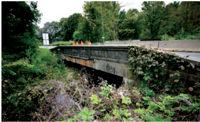
The Mill Street bridge over Washington Mountain Brook in Lee is visibly decaying. Replacing it will cost $8 million. Photo: Stephanie Zollshan, The Berkshire Eagle.
