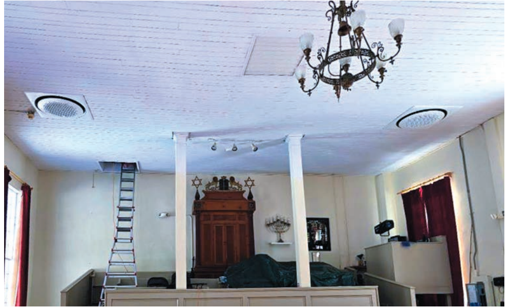
HVAC units have been installed in the ceiling of the main room.
