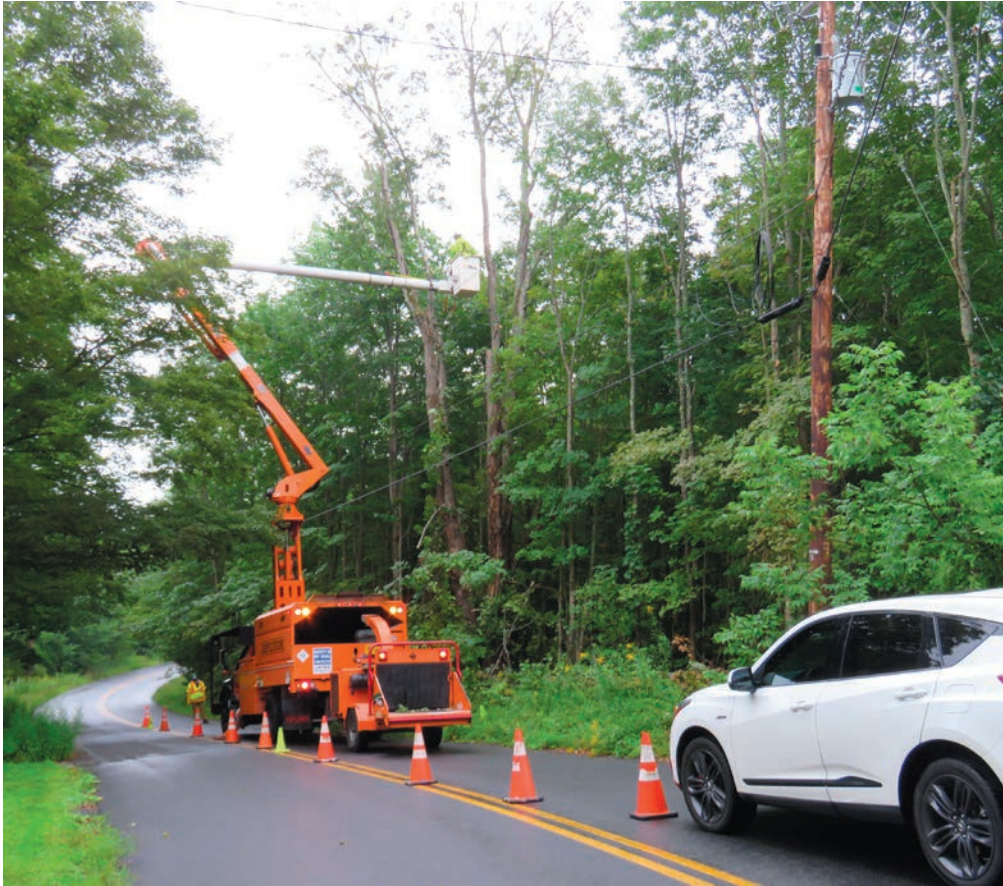
Crews worked through August and half of September in the Beech Plain section to remove trees deemed potential threats to the new broadband cables which were earlier installed several feet higher on poles.
