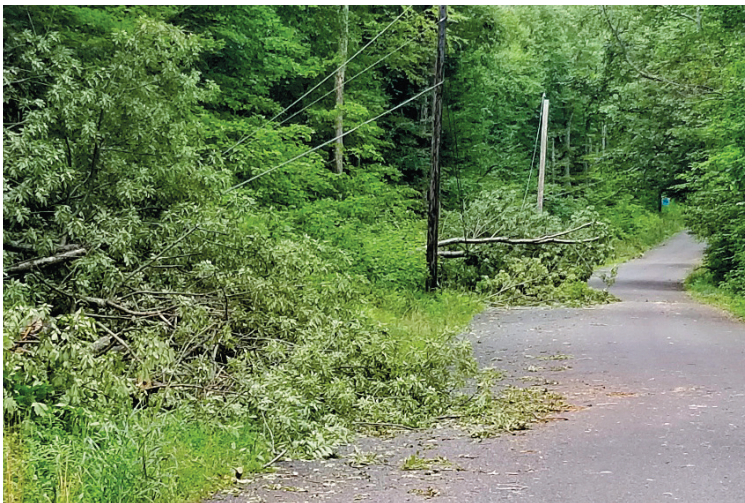
Power lines sag under the weight of fallen trees on Town Hill Road.
