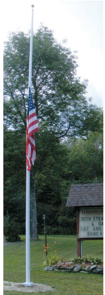
The new 35-foot flagpole at Firehouse #2, donated by a family that prefers to be anonymous. The pole was installed gratis by C.W. Nelson.
