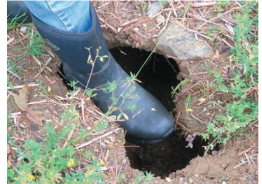
One of the series of sinkholes that have appeared near the pipeline.
