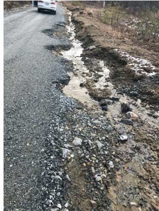
Dodd Road drainage. Without rip-rap, water is uncontrolled and erodes the road.
