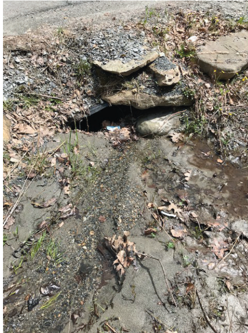
Clogged culvert at Dodd and New Hartford Roads. Unmaintained culverts pond up the water and undermine the road bed.
