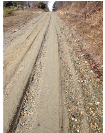
Dodd Road, last year. Without a crown and no drainage ditch, water drains down wheel tracks eroding road and softening roadbed. Mix of small rocks and fines do not compact or cohere so when wet it turns to mush.
