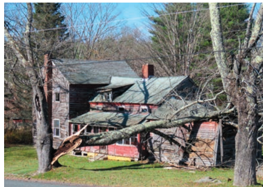
A storm in early November brought down the limb of a large tree onto the shed section of the red house, across Cold Spring Road from the barns.
