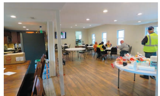
During and After. The new training center with renovations in progress, February 2017, and as recently completed.
