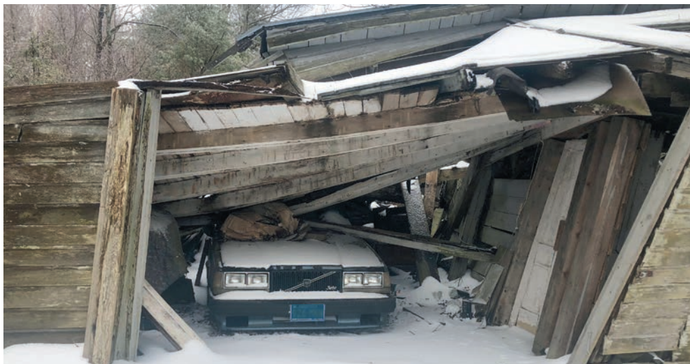
The View From the Road A barn that has been collapsing for several years at J. Jorgenson’s property on New Hartford Road has claimed another winter victim – a car that has been parked there since before the roof started to come down. Photo: Brigitte Ruthman
