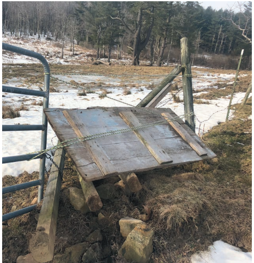
Stop-gap, but fixed for now.
