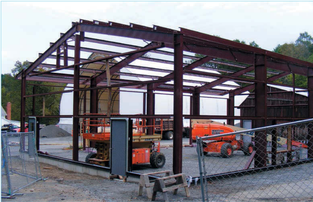
By the end of September, the concrete foundations had been dug and poured and the steel framework erected. The new garage is a bit larger, with bays on the side rather than the end of the building. BETNR Construction of Pittsfield expects to finish their work in about two months.
