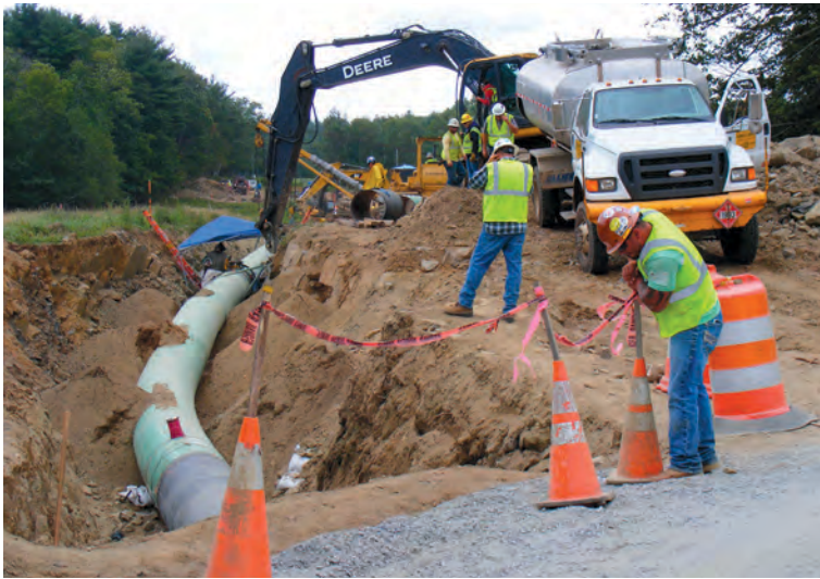
During Burying the pipeline on the east side of South Beech Plain Road.
