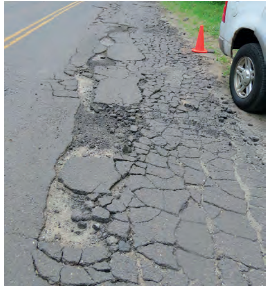
Deteriorating Cold Spring Road.
