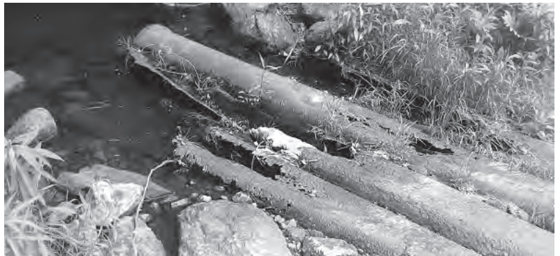
Pipes, now rusted and crumbling, piled across a pristine stream to serve as a “crossing” within what is now Spectacle Pond Farm. The makeshift bridge is still in place decades after the 1982 construction. Photo: Jean Atwater-Williams
