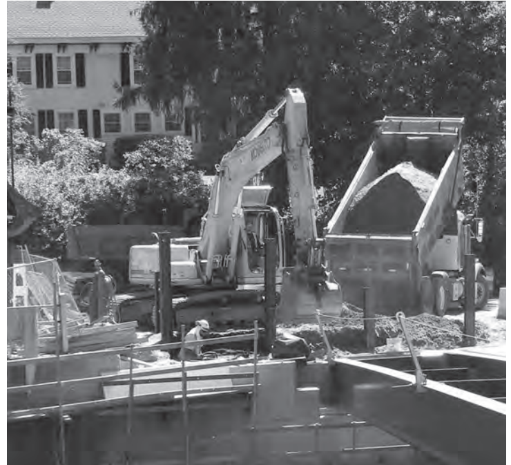
A JHM truck unloads sand at the bridge abutment by Tannery Road. JHM explained that construction of this section took longer than anticipated due to the number of large rocks encountered. Much of the work occurred directly in front of the former New Boston Store. Photo: Bill Price
