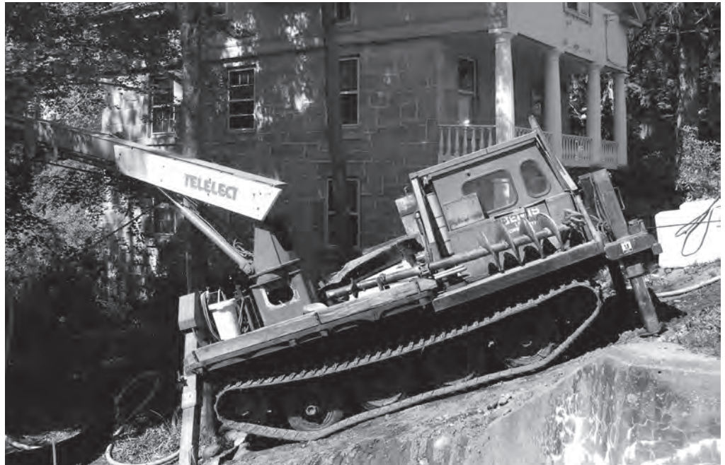
A roller-bit drill attached to a bulldozer was necessary to punch a hole next to the Old Stone House.
